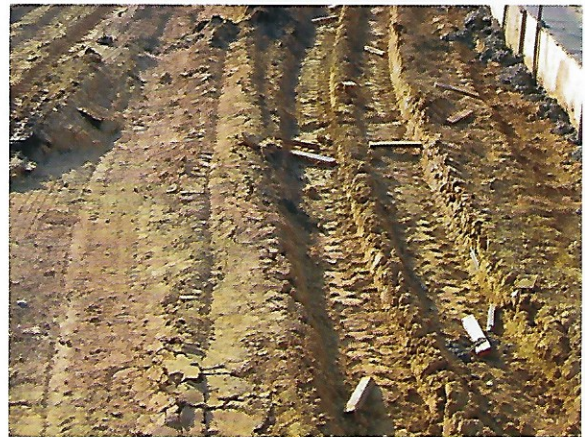
Example of failed sub grade
